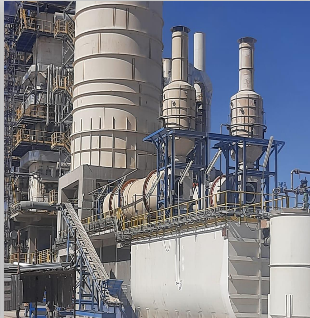
Lime Kiln station equipment “Biggest in the world” 11 conveyors + 2 lime slaker +4 vibrating screens / feeders
