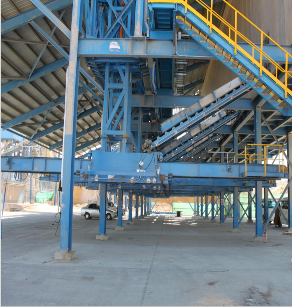
Bagging conveyors (8 bagging Lines) 8 intermediate conveyors 8 Telescopic conveyors
