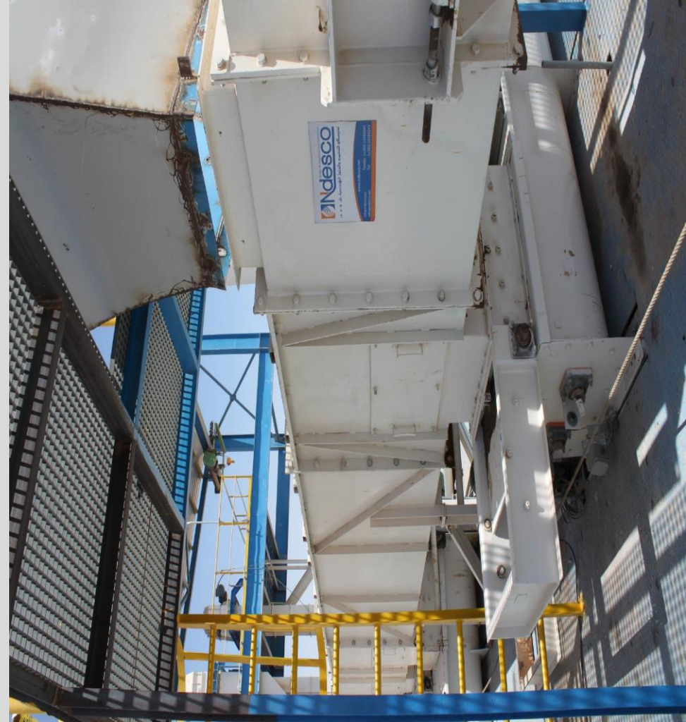
Pelletizing station Slide Gates – 5 Equipment
