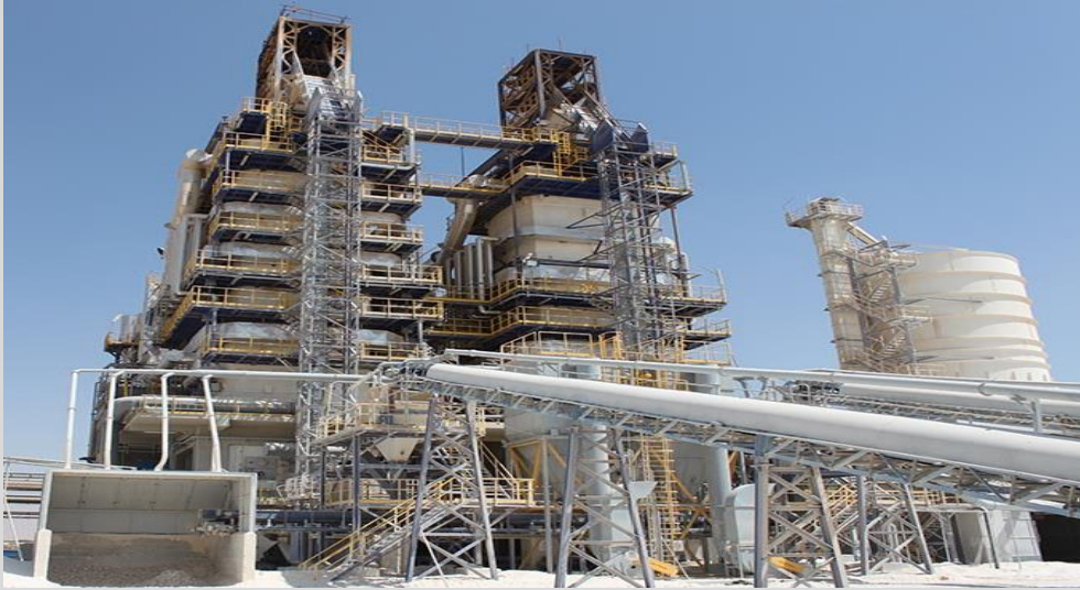
Lime Kiln station Belt Conveyors Qty. 11 Equipment
