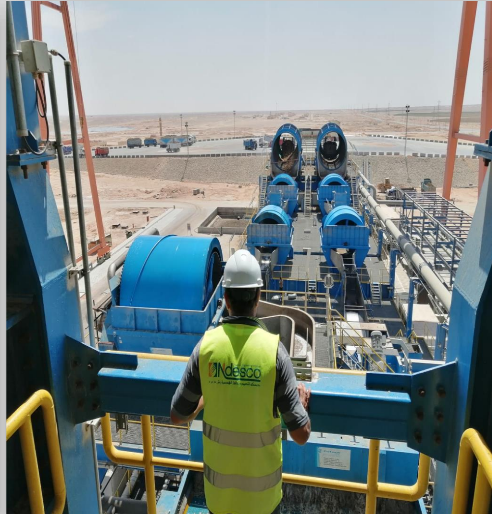
Washing station “Biggest in the world” Width 37m X Length 90m
