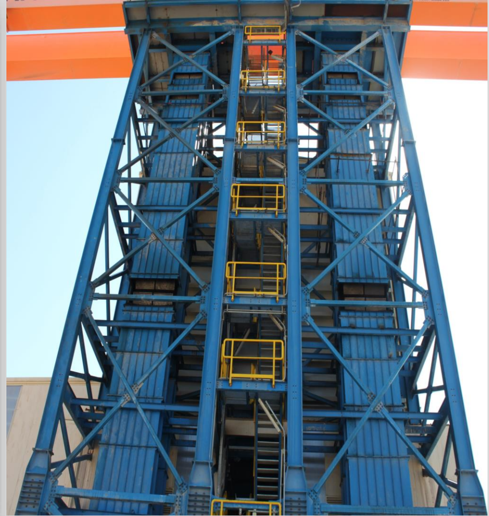
Clean beet bucket elevator “Biggest in the world” Capacity 1,500 Ton / Hr.
