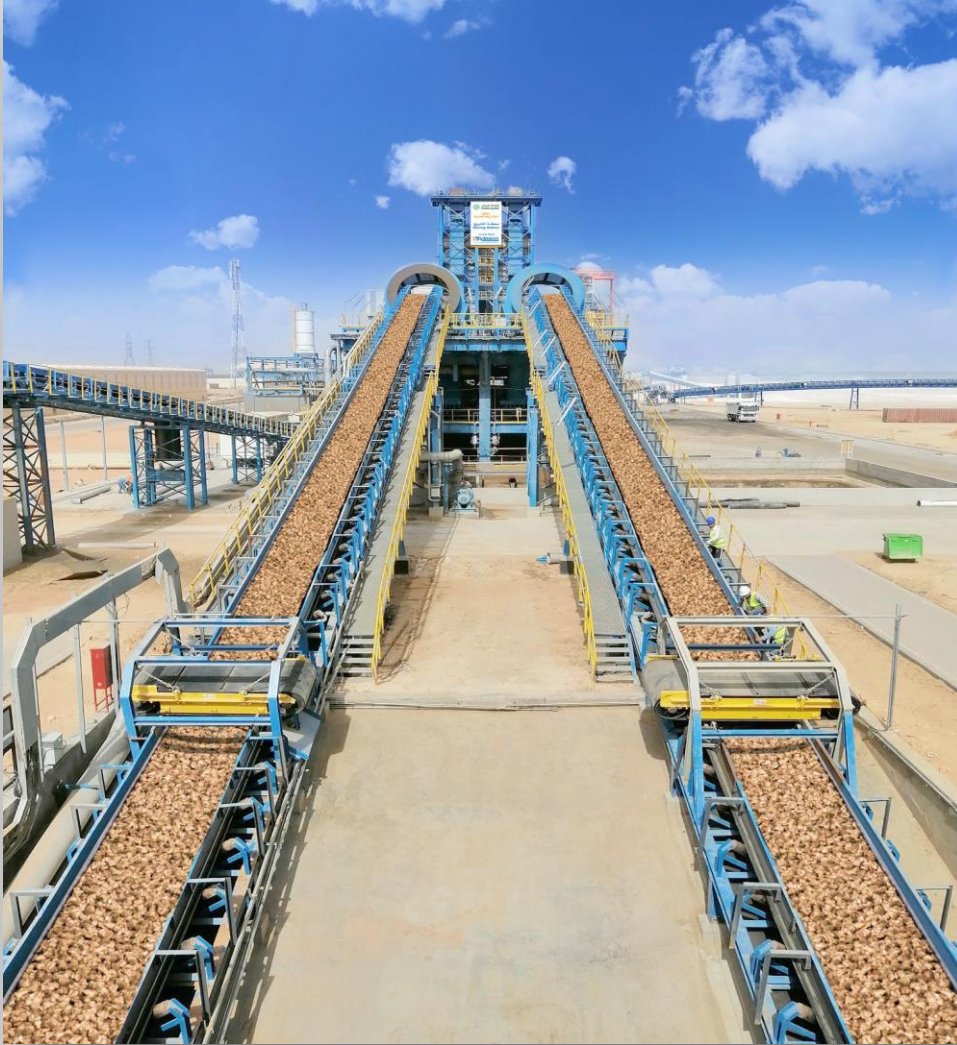
Dirty Beet Conveyors (Qty.2) Capacity 1,500 Ton / Hr.
