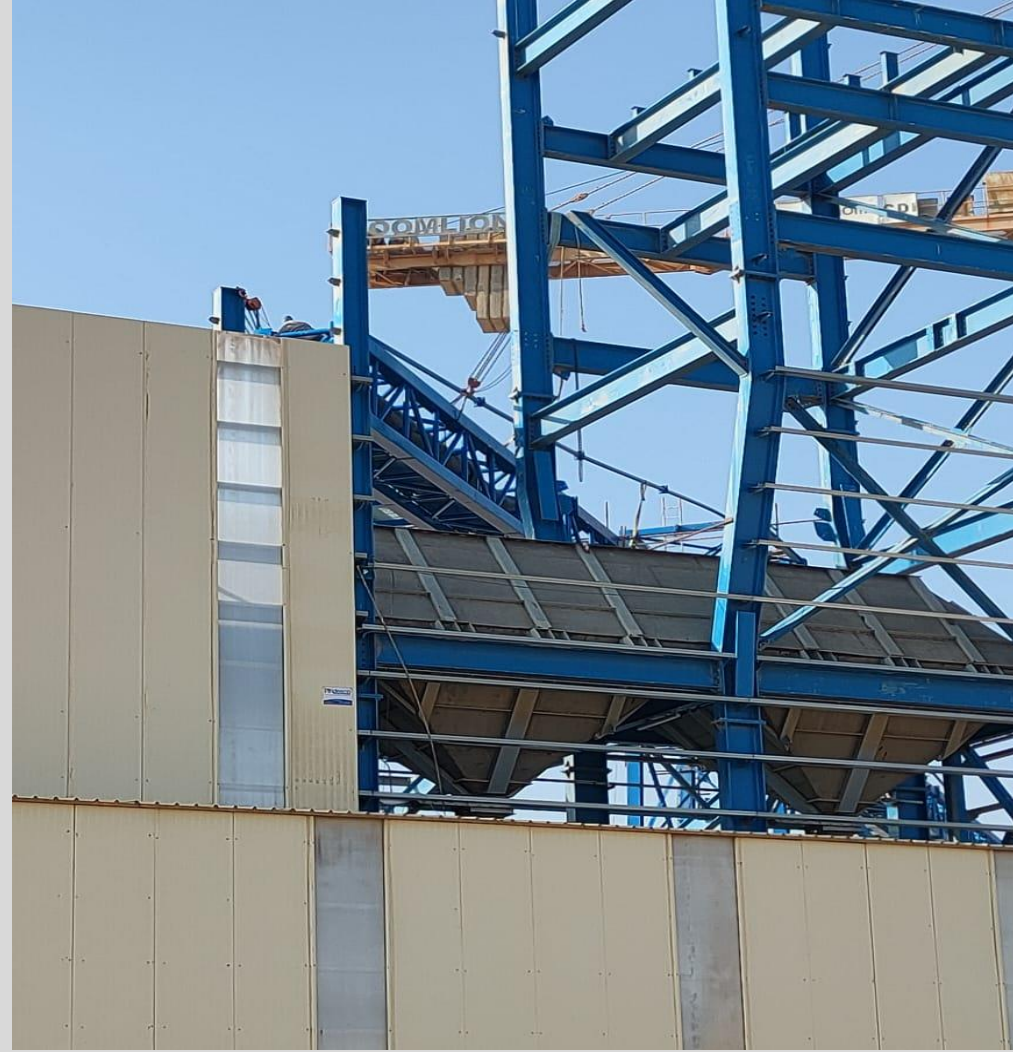
Final Sugar Bagging Hopper – L =48 m, H = 4.5 m
